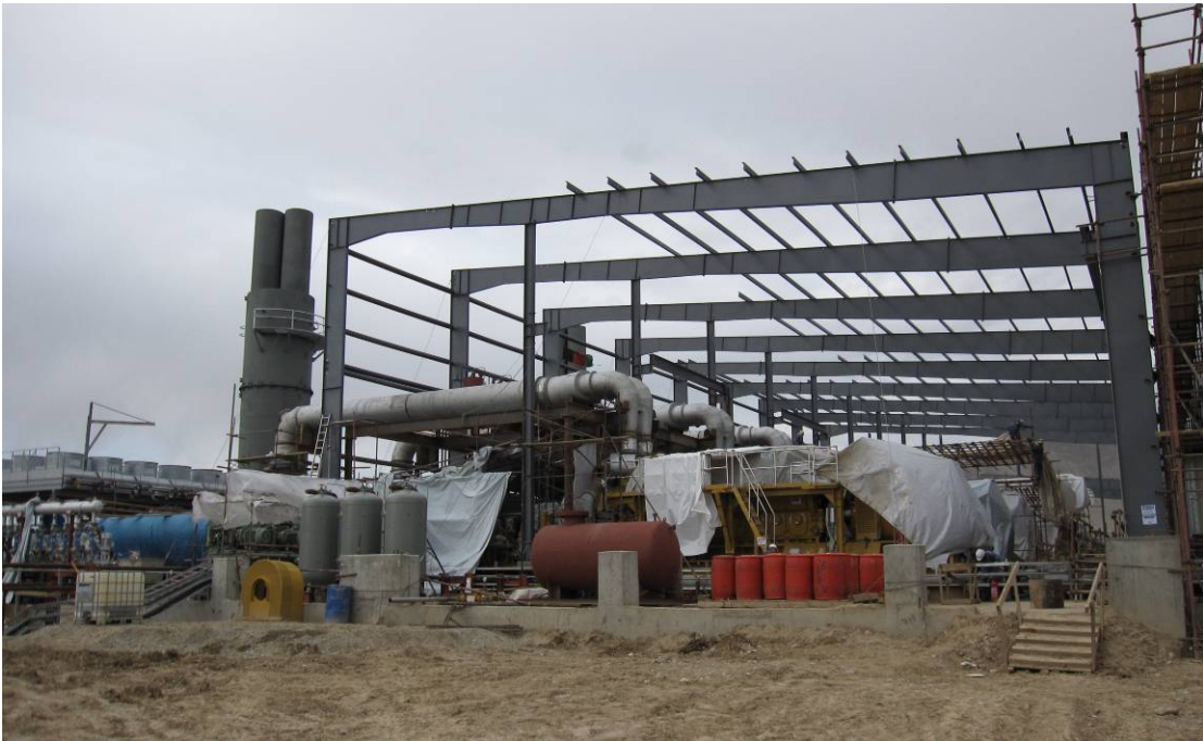
One of the generator blocks under construction in Kabul. (Photo by the Office of Inspector General, April 2009.)
