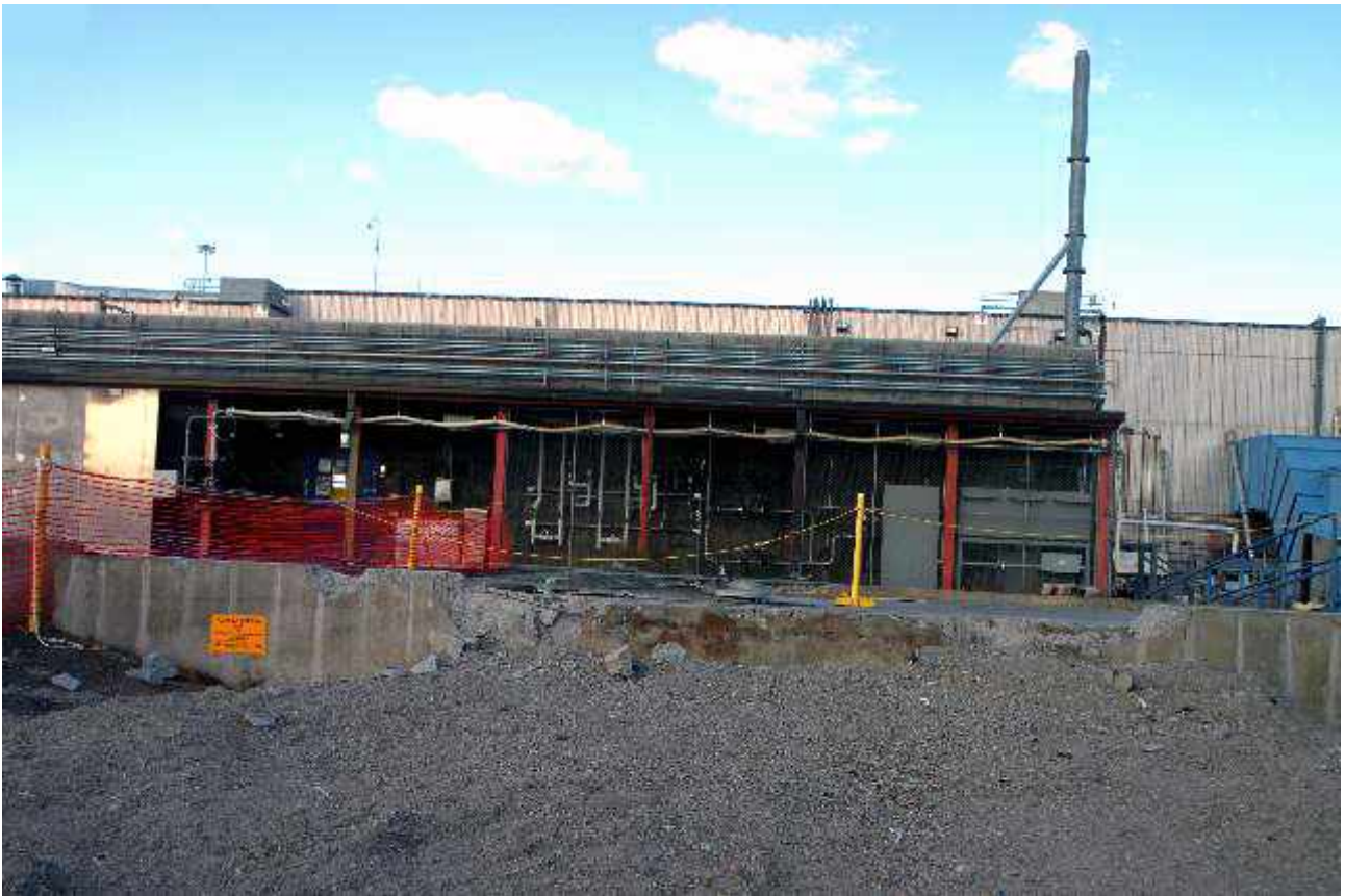
Demolition of Plutonium Vaults. Demolition is complete on building 2736-ZC, a 1,539 sheet-metal structure built in 1983 that served as a Cargo Restraint Transportation Dock.
